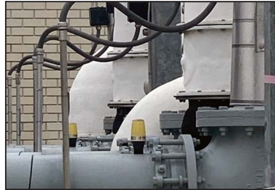
Submersible pumps with Chesterton Connect Sensors.
